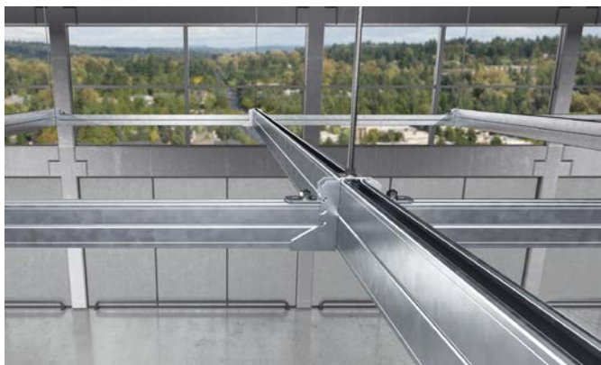
Installation grid in a production hall
